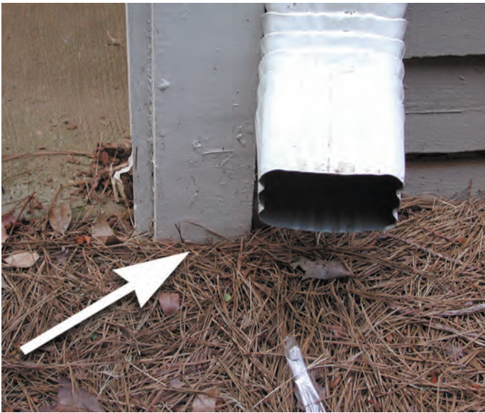
Figure 22. Wood to-ground contact (arrow) is a recipe for termite infestation. In this picture, wood is in contact with the ground in close proximity to where a gutter vents directly into mulch, resulting in persistently moist soil. Note also mulch piled next to the structure's siding
